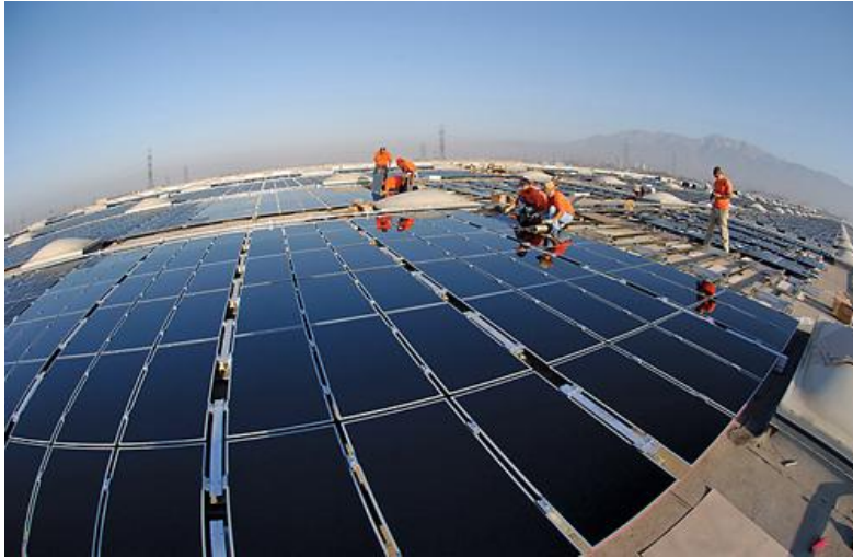
Many of the new green jobs in California are related to solar energy. Southern California Edison has several solar panel projects on top of distribution centers.
